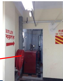
Boiler on 1 st floor
